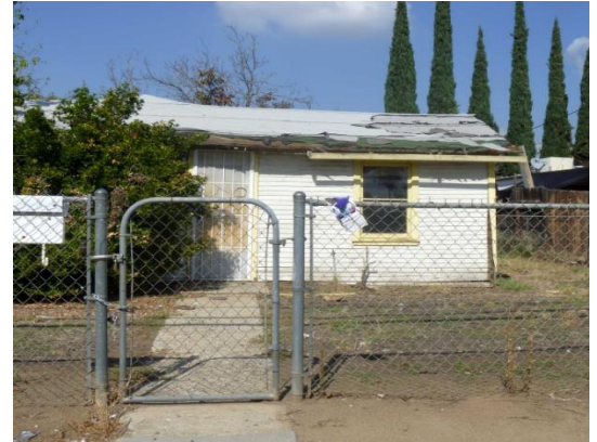
Example of Arvin Housing in Dilapidated Condition
