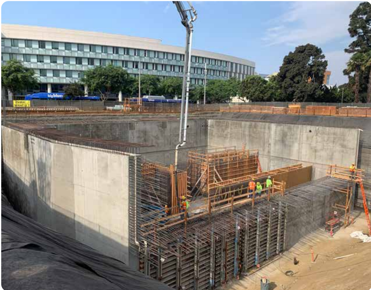
The stormwater and sewer treatment facility at the Civic Center Lot, part of the City's Sustainable Water Infrastructure Project (SWIP).
