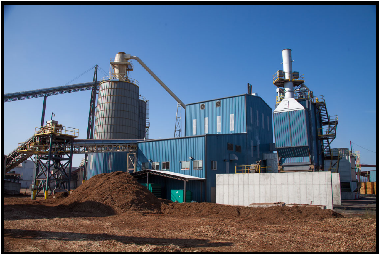
Figure 4.1A – 3 MW Boiler/Steam Turbine Cogeneration Power Plant
